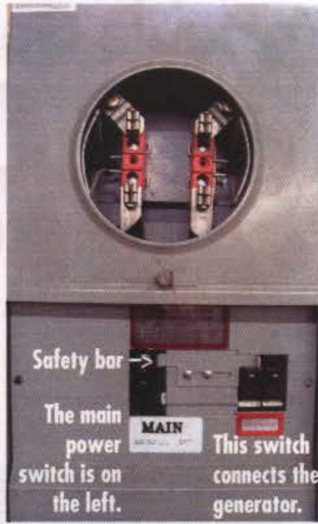
In this photo, the safety bar, which is locking out the generator switch, prevents backfeeding to the power lines.
